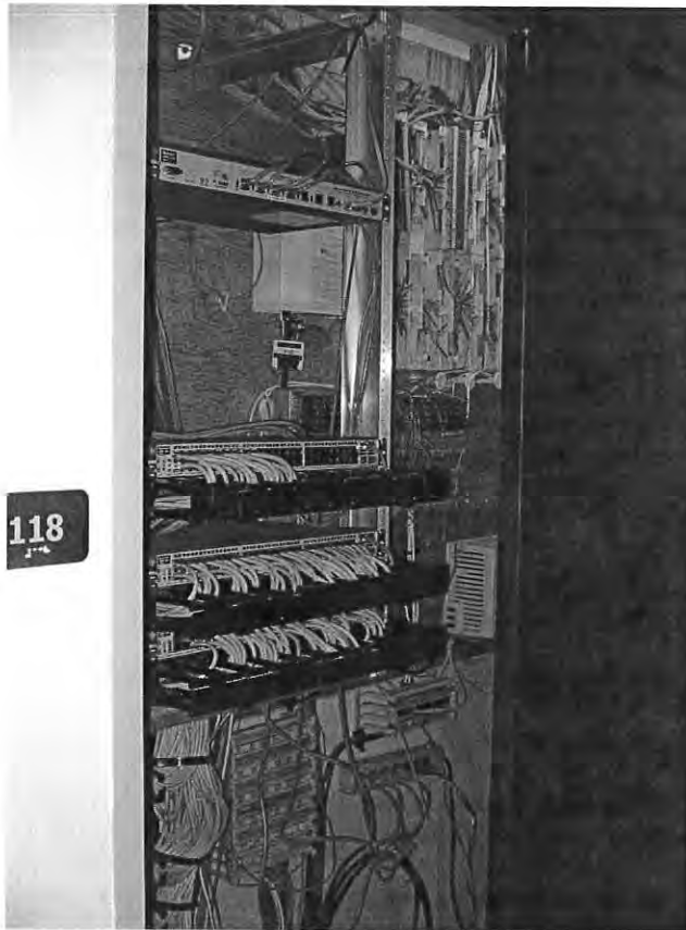
Unsecured and cramped closet at Owens Hall
