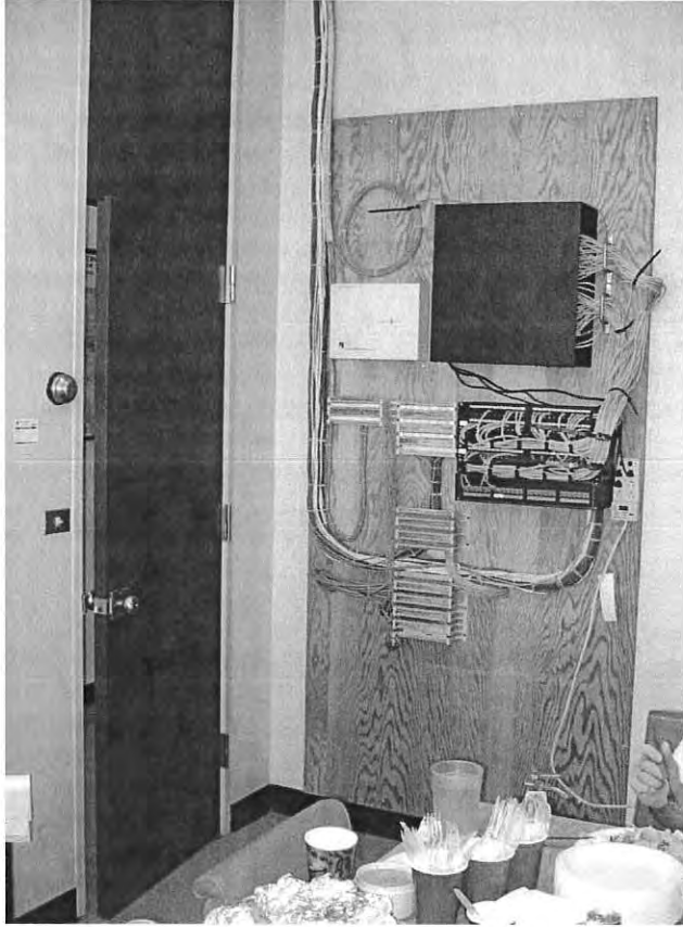
Unsecured Closet at Semon Hall
