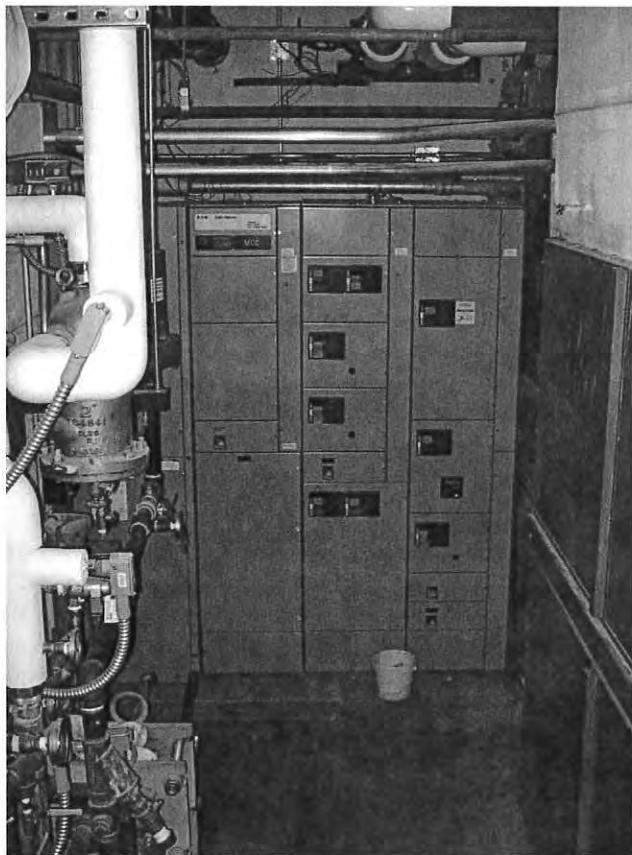
New Electrical Service for Point of Presence
